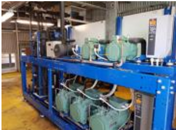
Figure 10 The CO 2 Transcritical Refrigeration Machinery
