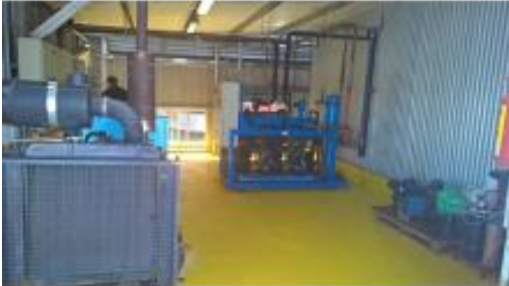
Figure 3 Baseline machine room
