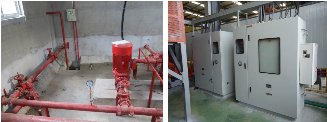
Fire equipment and anti-explosive control cabinet
