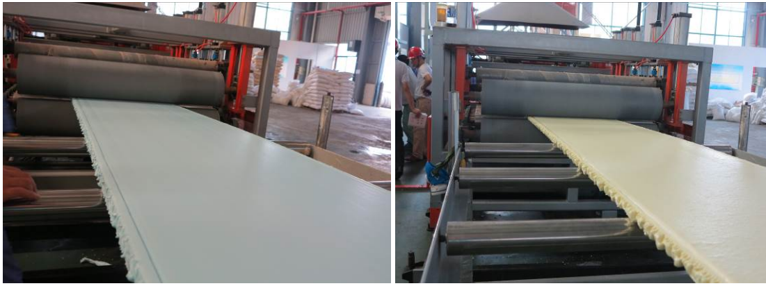
Commissioning/Trial-production by use of the CO 2 /Methyl formate co-blowing agent
