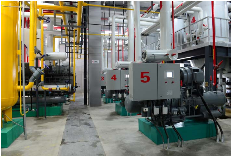
Fig 15. Running NH 3 /CO 2 system in customer
